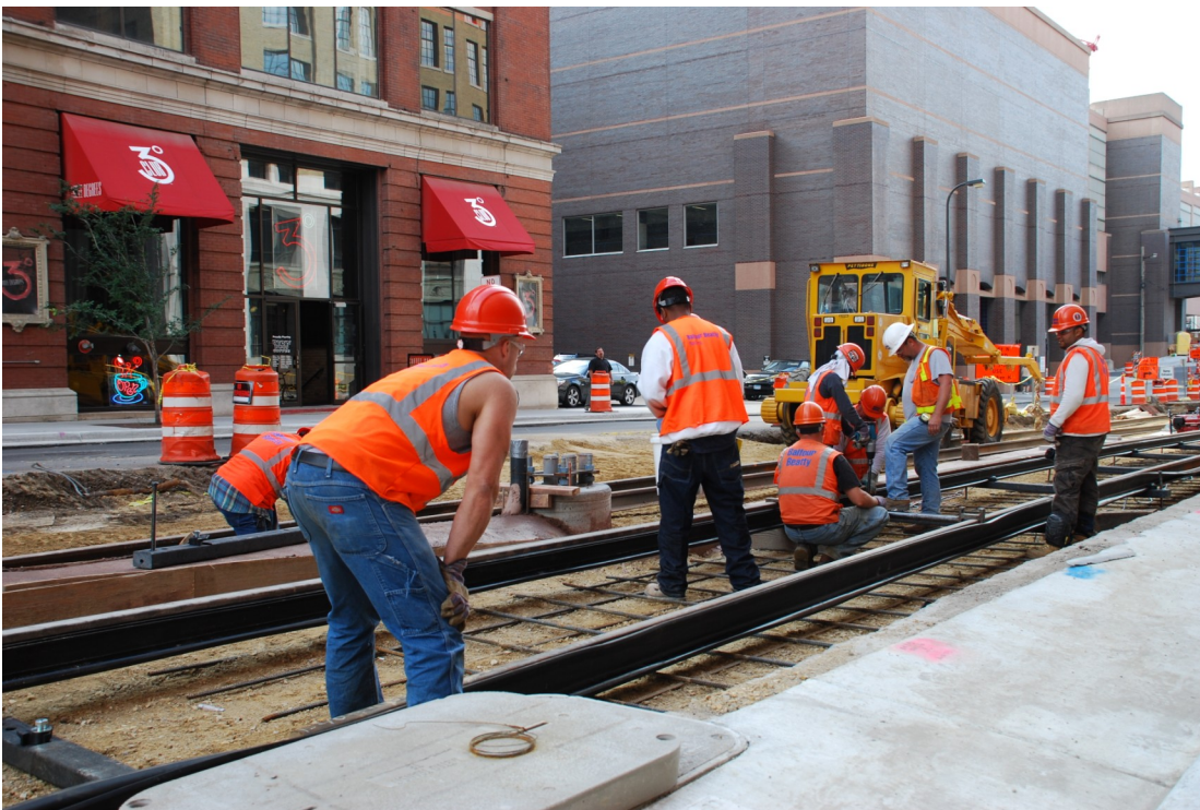
Crews place rail for embedded track for the Hiawatha LRT extension in downtown Minnea-
