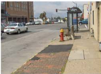
Streetscape shows signs of inconsistent repair and maintenance.
