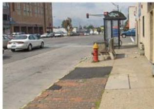
Streetscape shows signs of inconsistent repair and maintenance.
