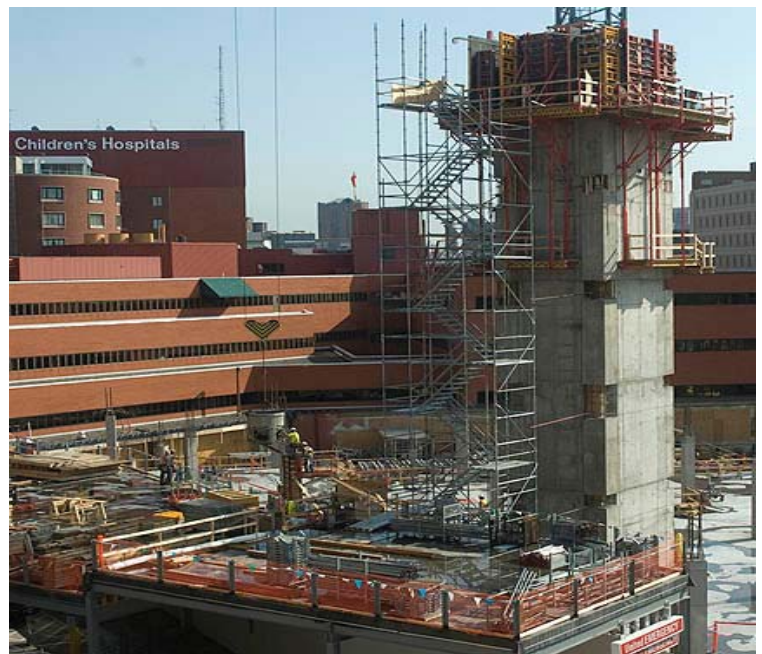
Children's Hospital expansion underway in downtown St. Paul. Photo by Metropolitan Council.
