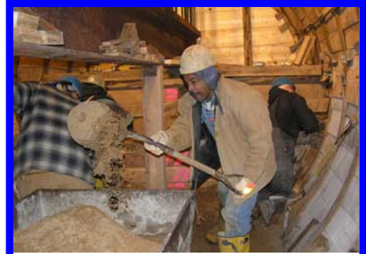
Empire Plant outfall. Hand-mining and reinforcing walls at head of a tunnel.
