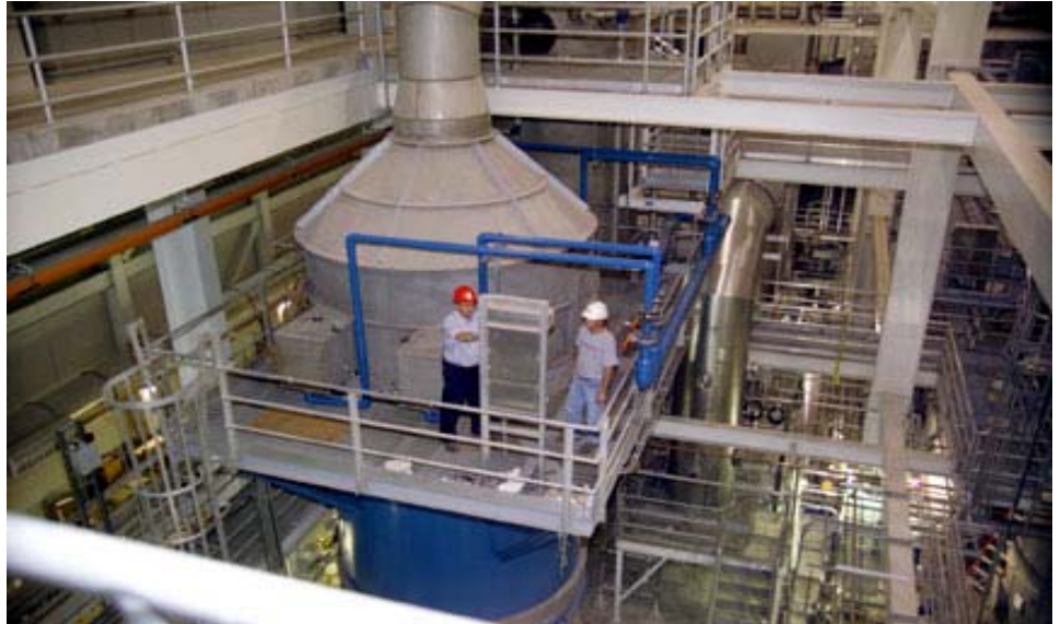
Plant operator Steve Harrom, left, and assistant business unit manager Tony Rudh monitor the early performance of one of the Metro Plant's new incinerators.
