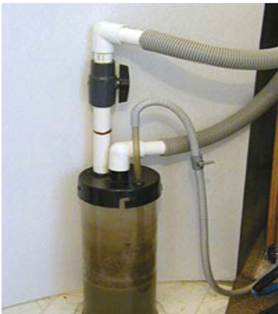
One of several approved amalgam separators in use at a dental clinic.
